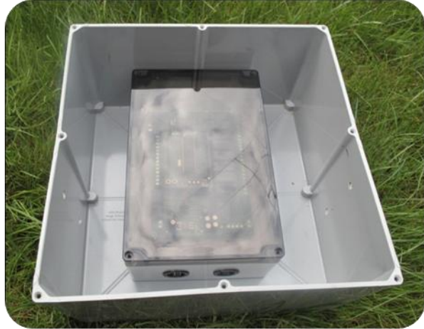
Relay Board mounted inside a Hammond watertight box inside a Home Depot watertight electrical box
